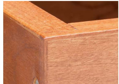
▲ The thin strips of wood covering the exposed plywood edges of the drawers make the joint lines virtually disappear.
